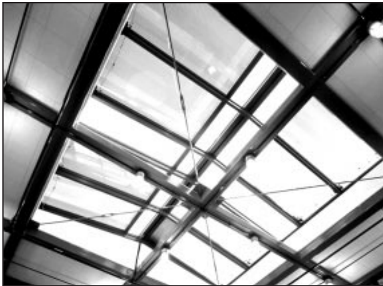
Fig. 4. PV skylight at APS facility, Fairfield, California. A standard skylight framing system mixing amorphous silicon PVs with tinted laminated glass. The PVs transmit 5% daylight.
