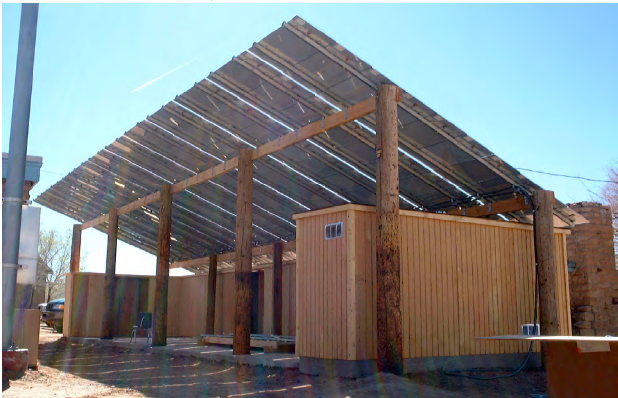
Seba Dalkai School, Seba Salkai, AZ. A K-12 school developed a solar curriculum to teach in this outdoor solar classroom..
