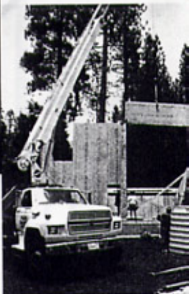
At noon, crane arrives to assist crew in placing large or high panels.
