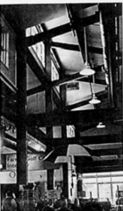
By exposing framework of Interbay Family Golf Center in Seattle, architect Jones & Jones achieved continuous SIP envelope.
