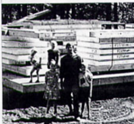
Bear Valley, California, architect David Wright (shown here with his four children) received delivery of SIP panels at 8 a.m.
